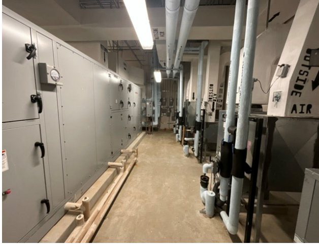
25 - AIR HANDLER AND HEAT PUMPS
