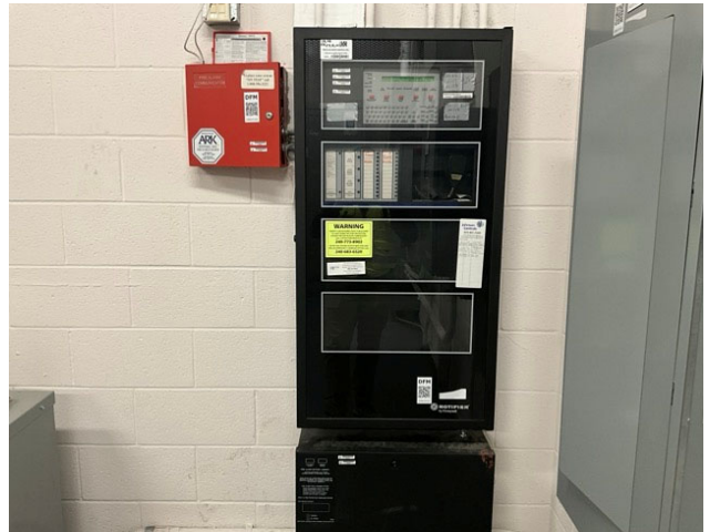
28 - FIRE ALARM PANEL
