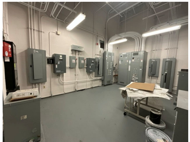
24 - MAIN ELECTRICAL ROOM
